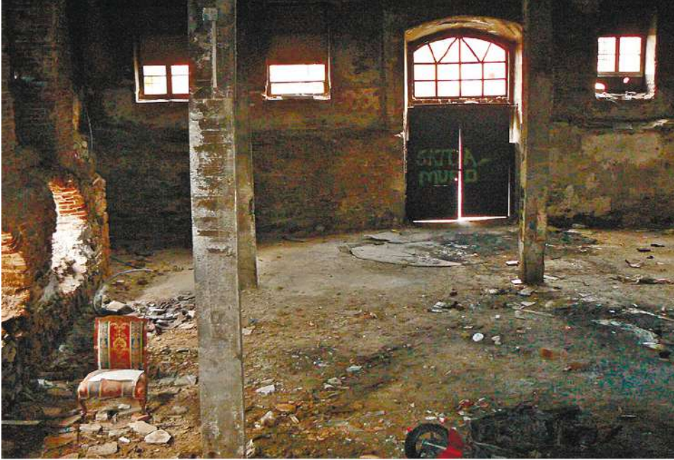
•The inside of the Khorenyan School. The school is now closed and nobody is allowed to enter. We were lucky that Romanos shared these photos, taken by him earlier.
